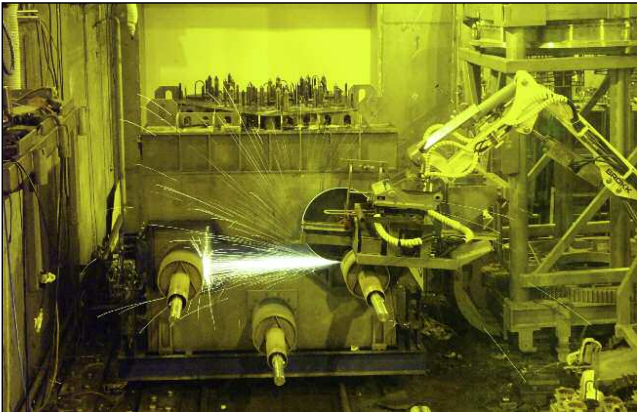
The Brokk, equipped with a circular cutoff saw, was used to cut the electrodes off the melter.
