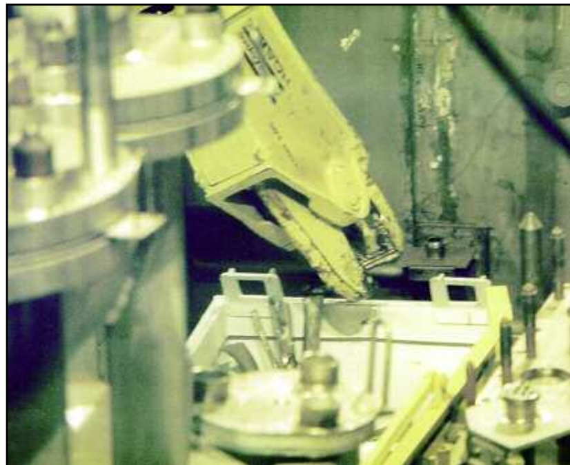
The Brokk, equipped with various end-effectors, proved useful during dismantlement of the vitrification cell.
