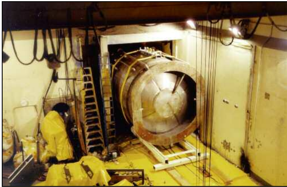
The CFMT is being drawn through the EDR shield door into the staged waste container.
